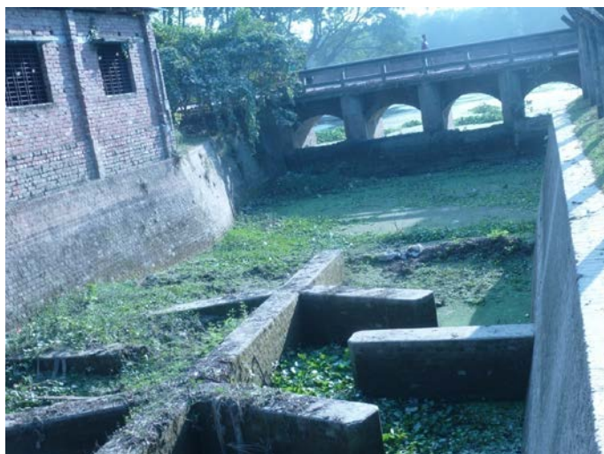
Photograph 3.1: The water regulator structure - fish by pass and sediment trap (British design) at the mouth of Kata Khal joining the Kobadak at Jhikargacha.
